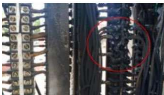
Gambar 4. Terminal Marshalling Kiosk Terbakar
