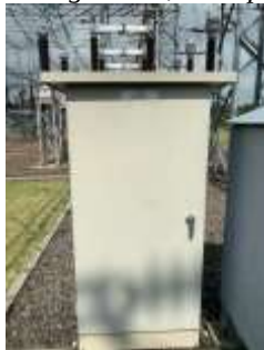
Gambar 1: Marshalling Kiosk Outdoor.
